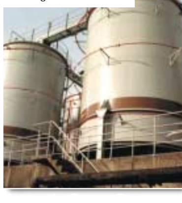
Holding Tanks & Bunds
